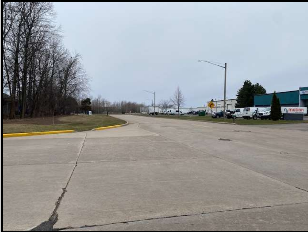
View of Kennedy Avenue, looking westerly from the intersection with Ford Street (Station 36)
