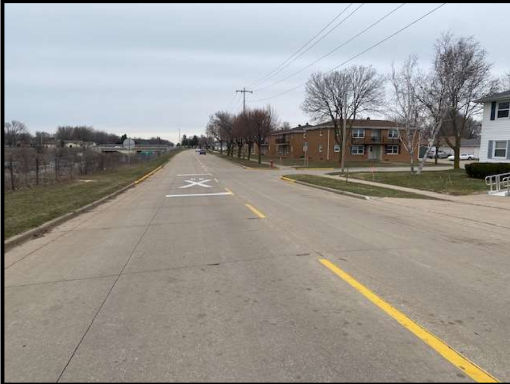
View of Marcella Street, looking northerly from near the intersection with West Fourth Street (Station 19)
