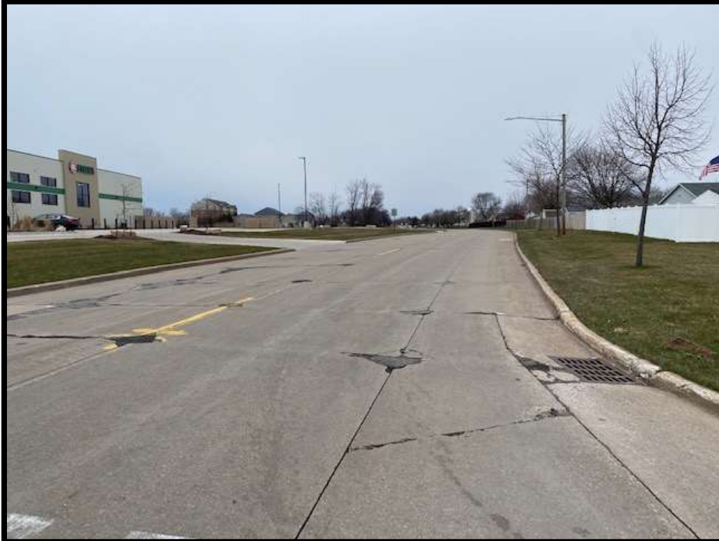
View of Kennedy Avenue, looking westerly from the intersection with Cobblestone Lane (Station 64)
